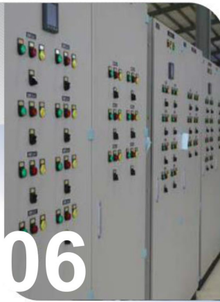
TỦ CP Control Panel (CP)
