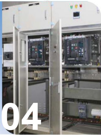
TỦ MSB Main Switchboard (MSB)
